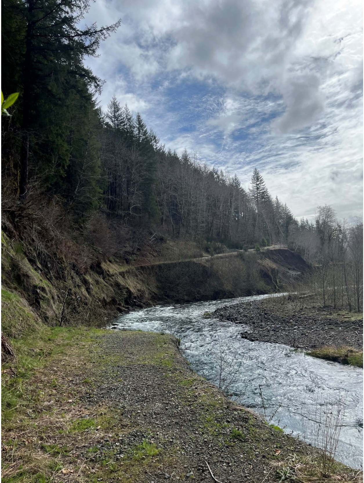
2 Photo of the section of Cook Creek Road that washed out into Cook Creek, image taken April 2023.
